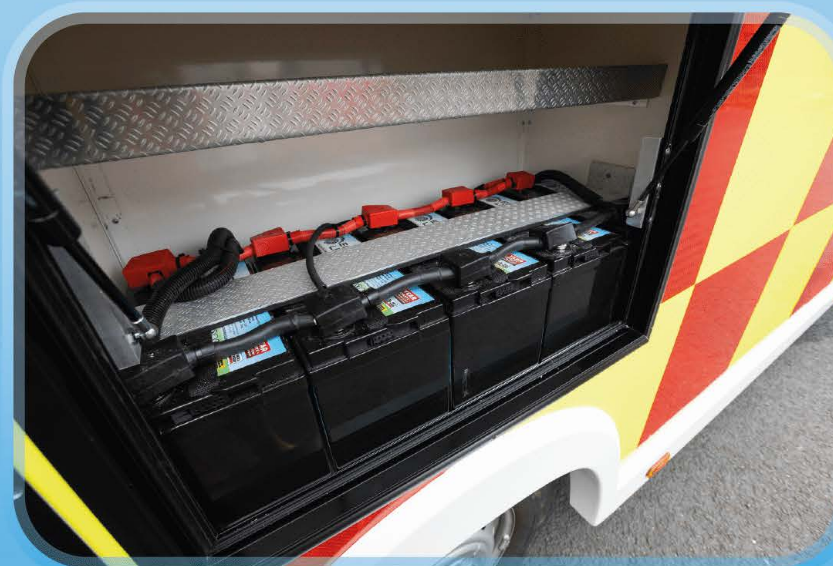
6 x 12.8v 100ah Lithium Iron Batteries
